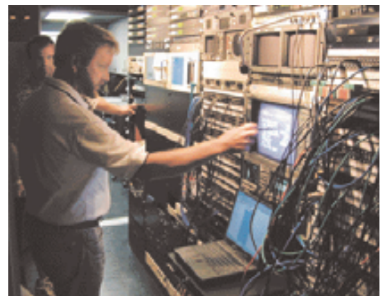
Marv White, Sportvision’s vice-president of engineering, checks monitor in RaceFX control center.
